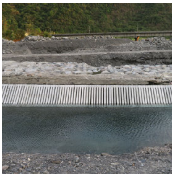
^ Fig. 5 The construction of the underground weir in EICS (Source: Szu-Ling Lin and Cheh-Shyh Ting).
