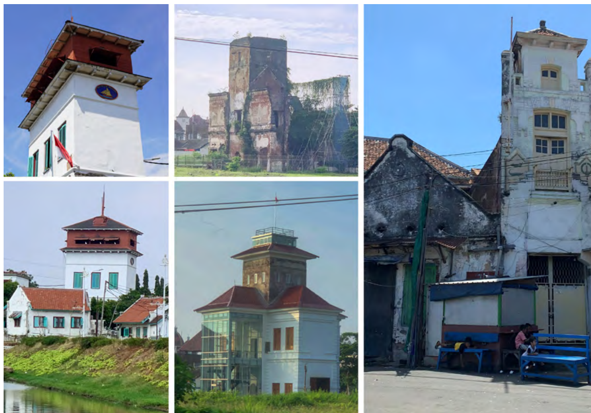
^ Fig. 3 Conditions of the three harbormaster towers: Batavia/Jakarta (after restoration, left), Semarang (before and after restoration, center), and Surabaya (current condition, right) (Source: Ricky Purbaya, 2024).
