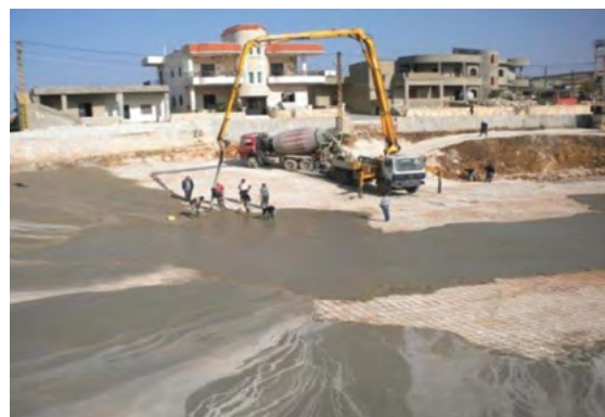
^ Fig. 3 Workers laying a steel-rod mesh with ready-mix concrete at the birket of Marwaheen (Source: American University of Beirut's Center for Civic Engagement and Community Service Report, 2013).
