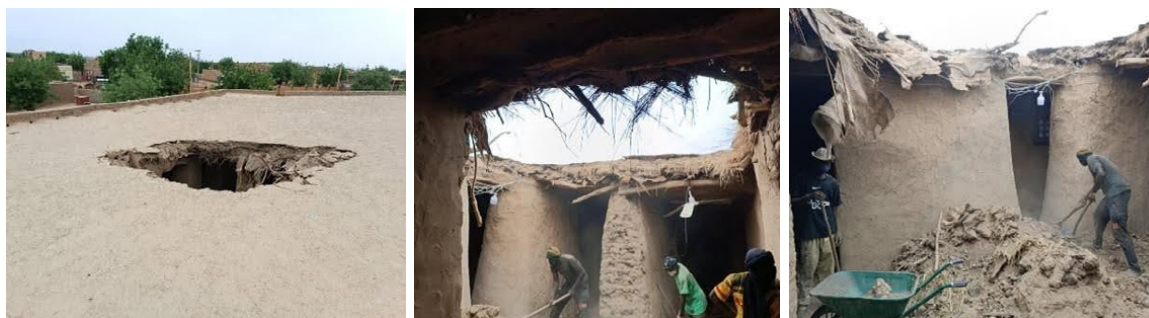
^ Fig. 2 Collapsed men's mosque roof (Source: Mamadou Samaké, 2024).
