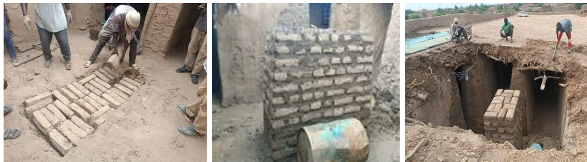
^ Fig. 3 Repair work on the roof of the men's mosque after the 2024 collapse (Source: Mamadou Samaké, 2024).
