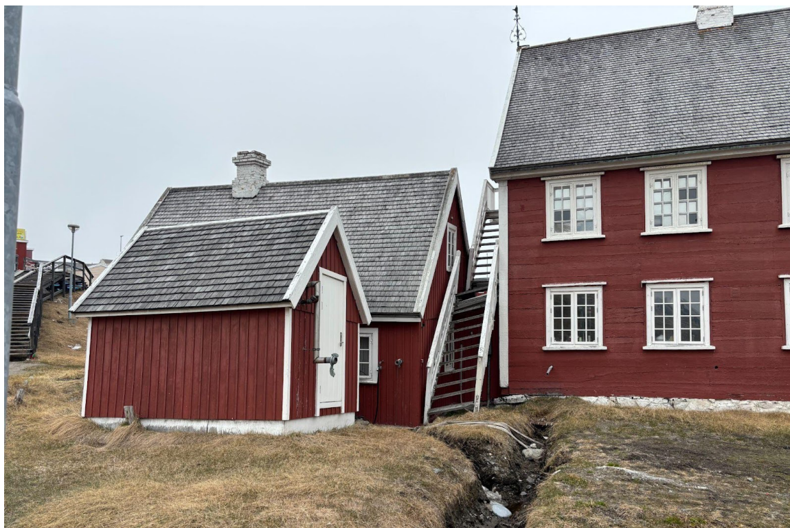
^ Fig. 2 The Ilulissat Cultural History Museum is sinking as thawing permafrost undermines its foundations (Source: Bo Albrechtsen, 2025).
