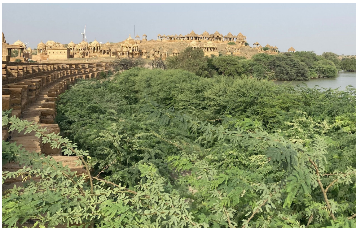
^ Fig. 4 Stone embankment overrun by vegetation at the Bada Bagh Khadeen (Source: Pierantonio La Vena, 2023).
