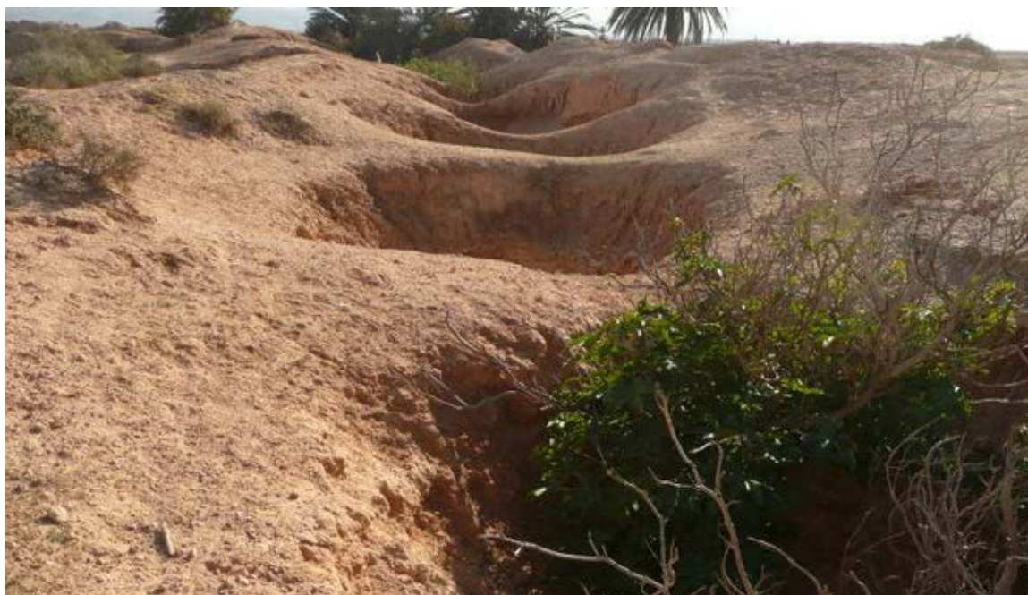
^ Fig. 4 The tops of khattara maintenance shafts with signs of dereliction and overgrown vegetation, threatening their collapse, Guelmim region, Morocco (Source: Cristiana Strava, 2010).
